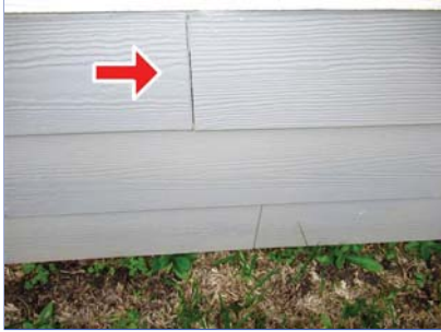
E. Item 2(Picture) cement fiber board joint
