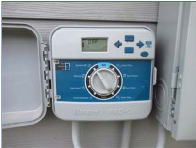
A. Item 1(Picture) sprinkler timer/ controller
