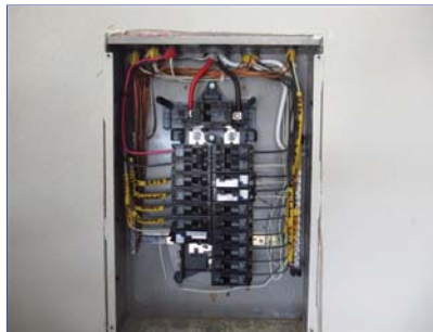
A. Item 4(Picture) sub panel - interior
