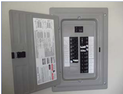
A. Item 3(Picture) sub panel
