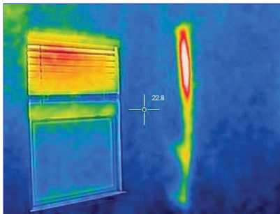
C. Item 4(Picture) bedroom wall behind water heater
