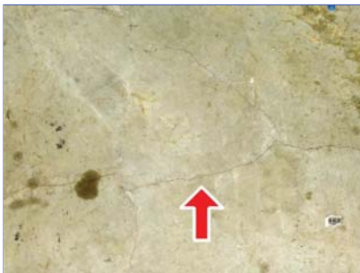
A. Item 1(Picture) curing cracking (garage)
