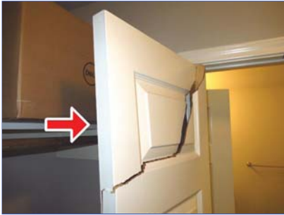
G. Item 1(Picture) broken closet door
