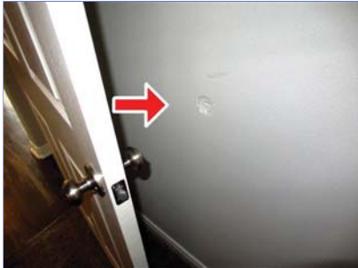
E. Item 3(Picture) door knob damage
