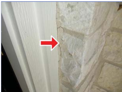
E. Item 1(Picture) mortar cracking
