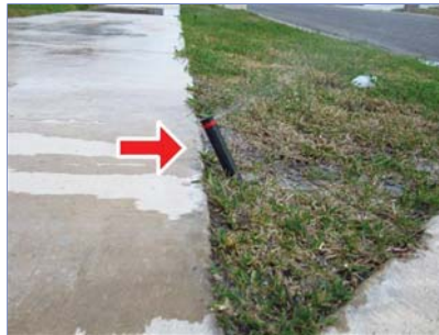
A. Item 4(Picture) not perpendicular to ground
