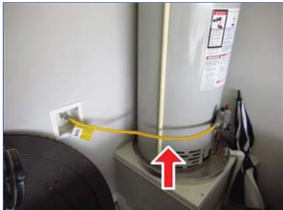
C. Item 4(Picture) missing sediment trap
