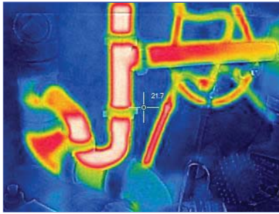
C. Item 2(Picture) kitchen sink drain
