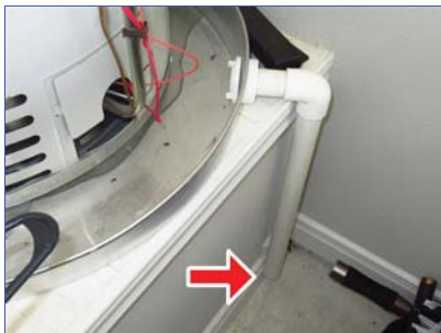
C. Item 3(Picture) drains onto garage floor
