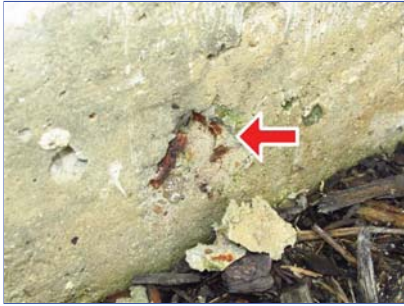
A. Item 2(Picture) exposed rebar (front flower bed)
