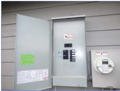
A. Item 1(Picture) main panel
