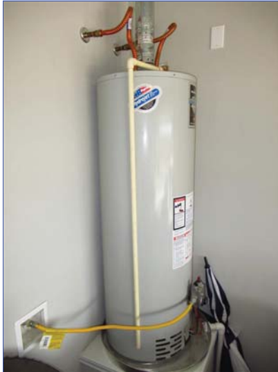
C. Item 1(Picture) water heater
