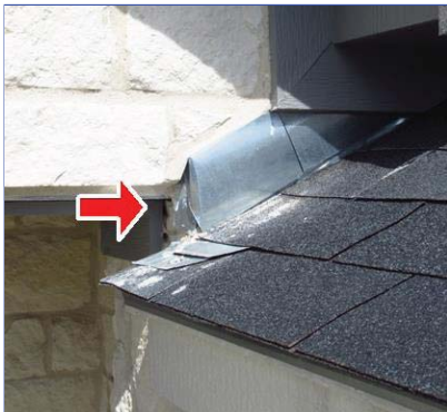
C. Item 3(Picture) missing kick out flashing
