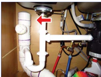
B. Item 1(Picture) missing AAV
